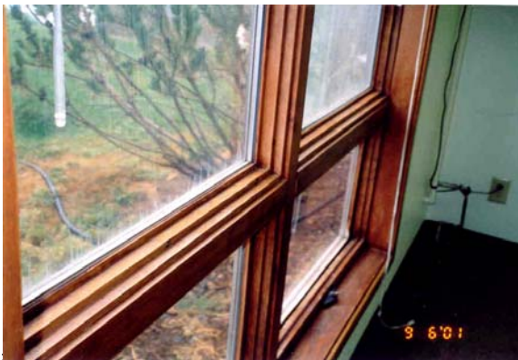
Example of IG Window Unit Failure: Note “streaking” on glass and “foggy” air space.
